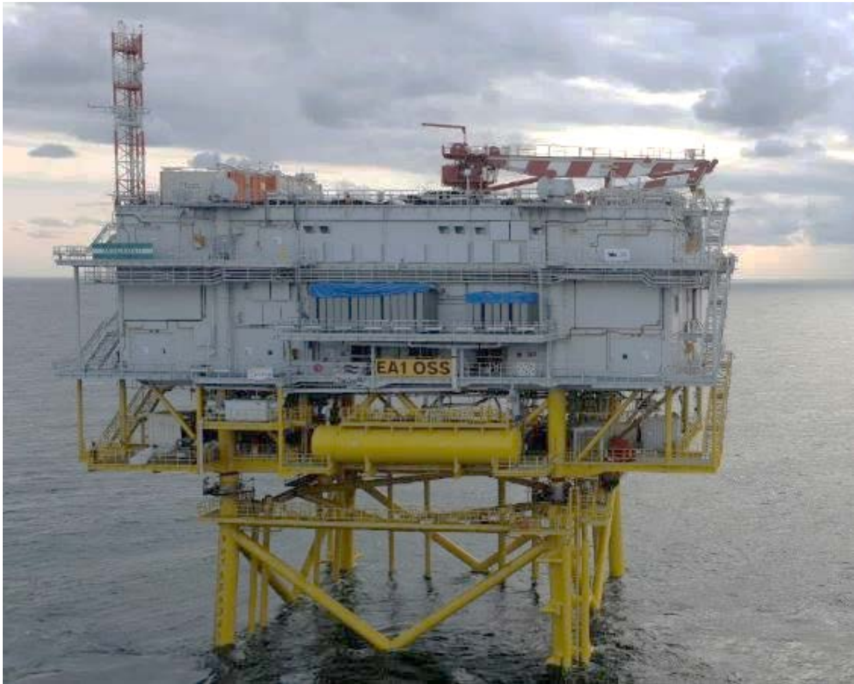
Plate 6.9 Typical offshore electrical platform (AC collector station)
