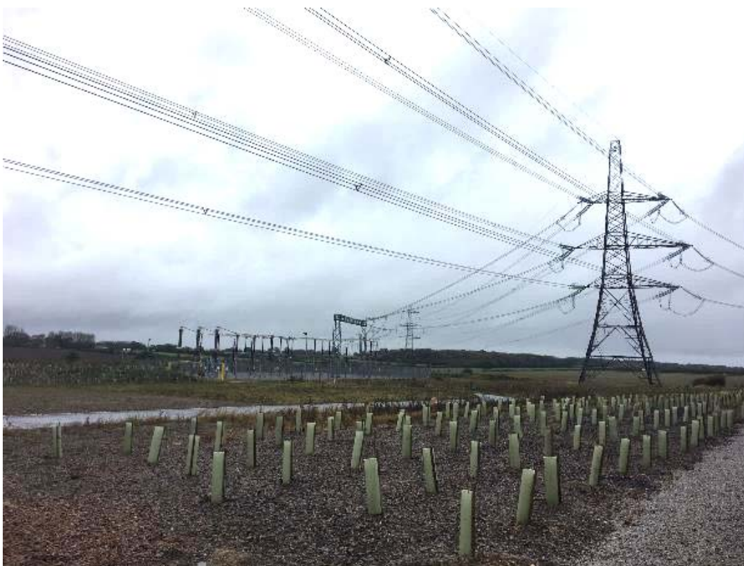
Plate 6.31 Example of Cable Sealing End Compound
