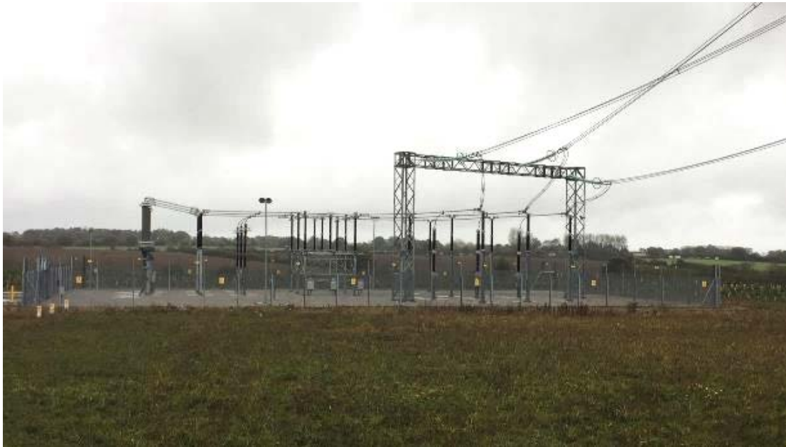
Plate 6.30 Example of Cable Sealing End Compound
